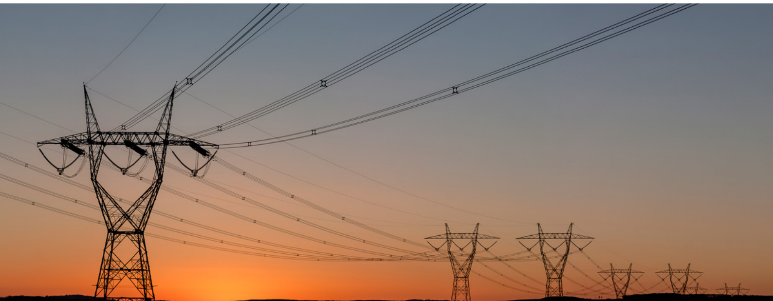
Figure 3: Extreme heat can have significant impacts on infrastructure and essential services, such as electricity transmission.
